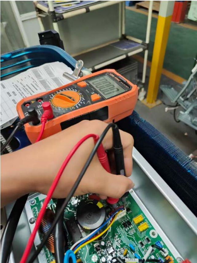
The multimeter measures the voltages of each wire sequence and the ground wire.
