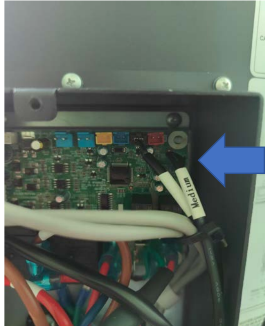
The temperature in the middle of the water tank corresponds to the TH1 PCB board of the water tank.
