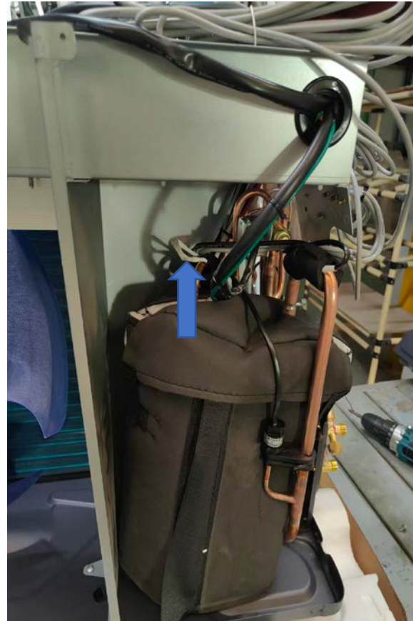
Discharge temperature probe position
